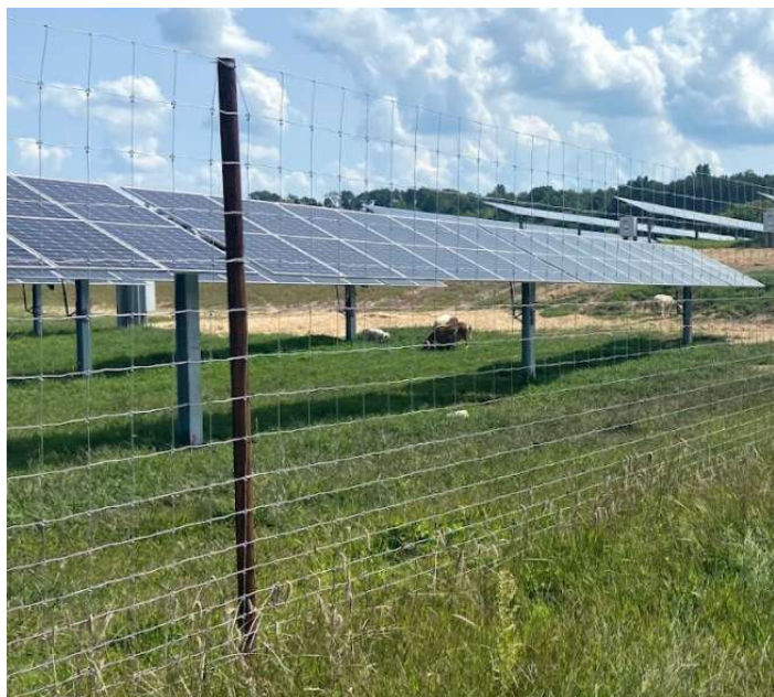
Fence at Rushford Village Solar Project in Rushford Village, MN
