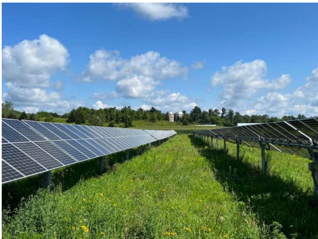
Strobus Solar Project in Black River Falls, WI
