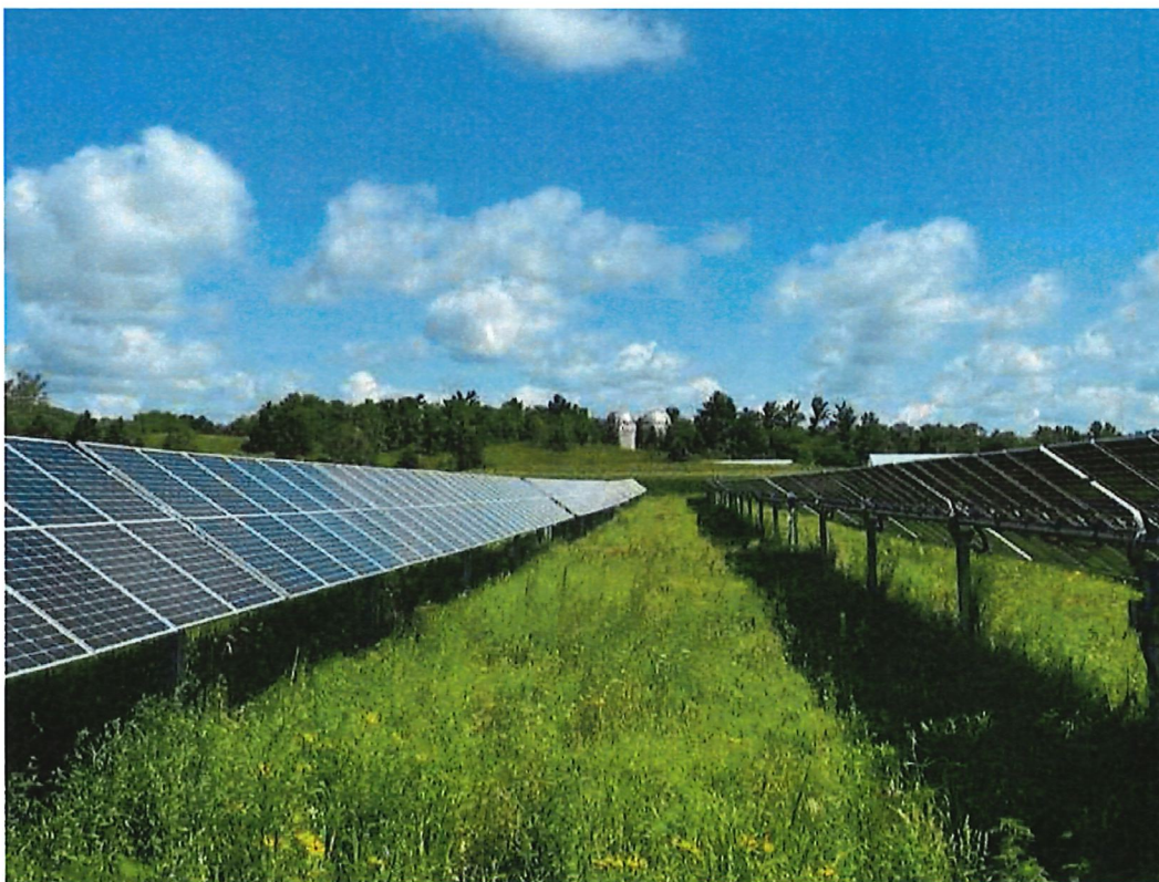
Strobus Solar Project in Black River Falls, WI
