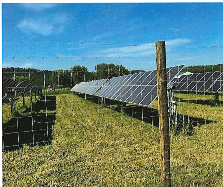
Fence at Blue Prairie Solar Project in Black River Falls, WI
