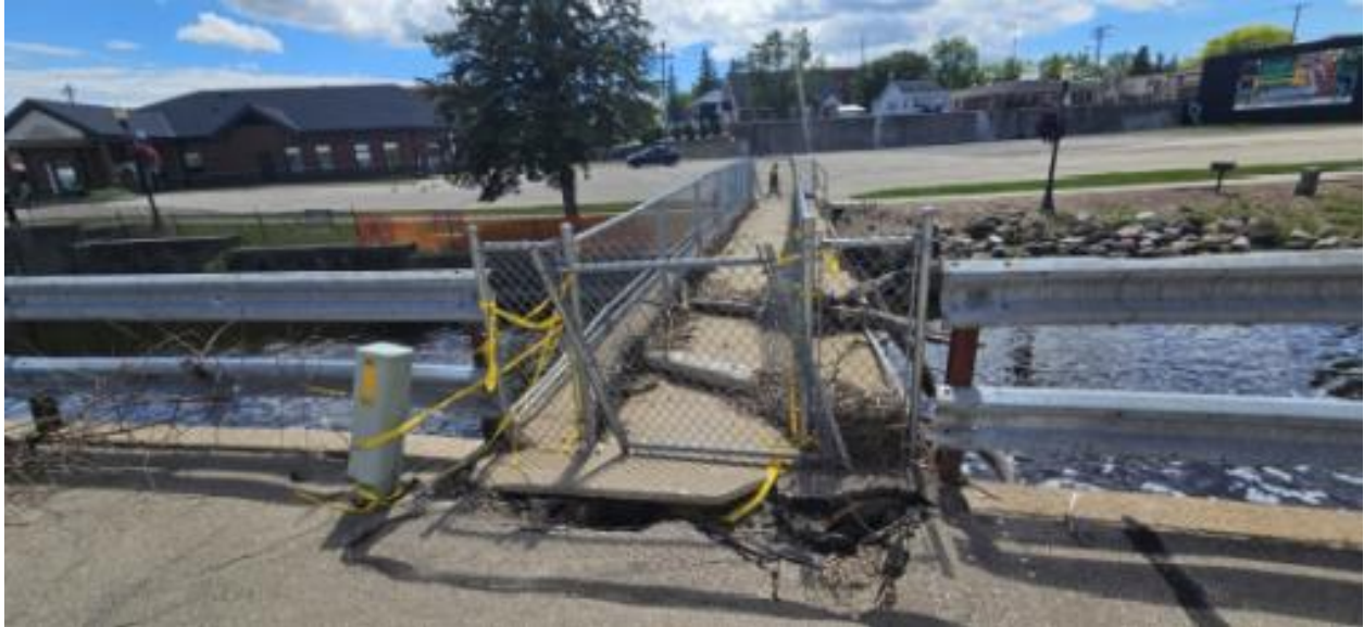
North side of Bridge showing washout over Retaining Wall / Abutment
